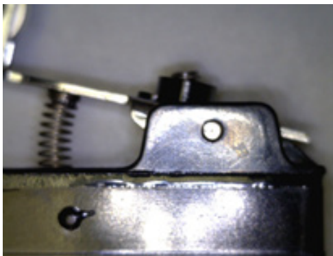
Figure 6. Example of Set Screw Misalignment Within the Eaton Switch
