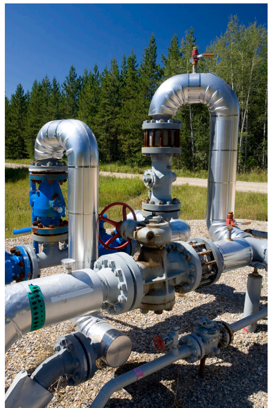
Figure 2. Flow Meter in a Gas Pipeline
