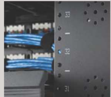
High-visibility full RU markings
