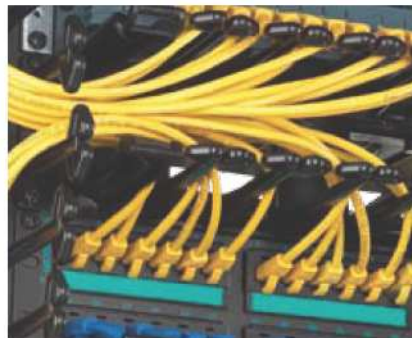
No sharp edges to damage cables.
