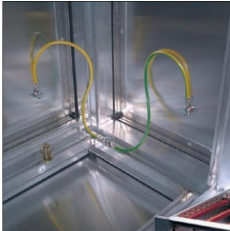
Earthing of removeable parts in a cabinet
